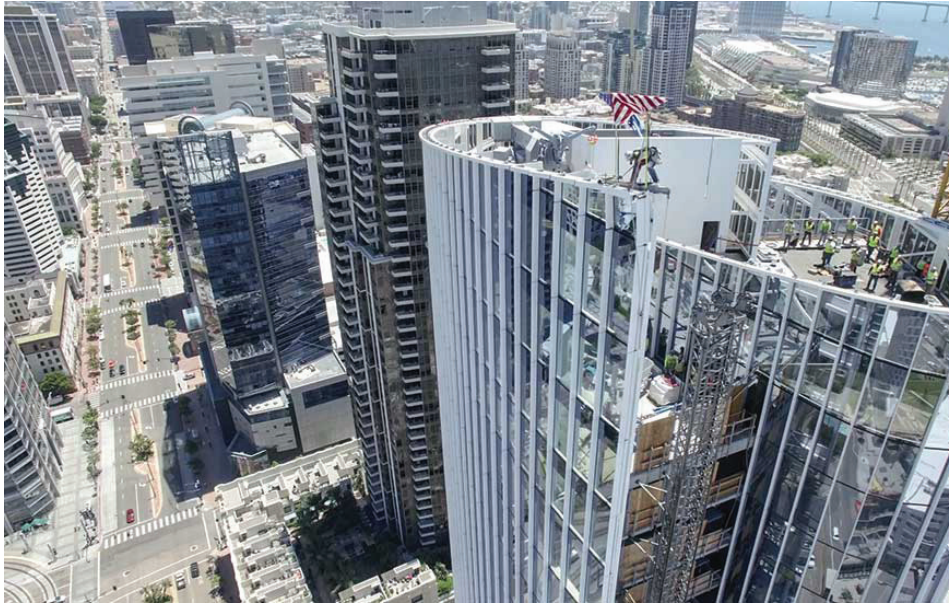
Enclos installed 320,000 sq ft of custom curtain wall and facade on Pacific Gate, a 41-story, 514,000-sq-ft luxury apartment building in San Diego. PHOTO COURTESY OF ENCLOS
